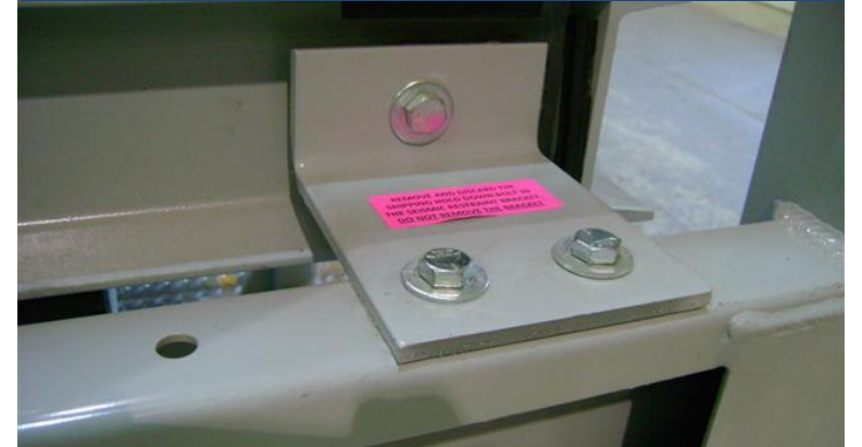
Seismic Restraint and Shipping Tie Down
